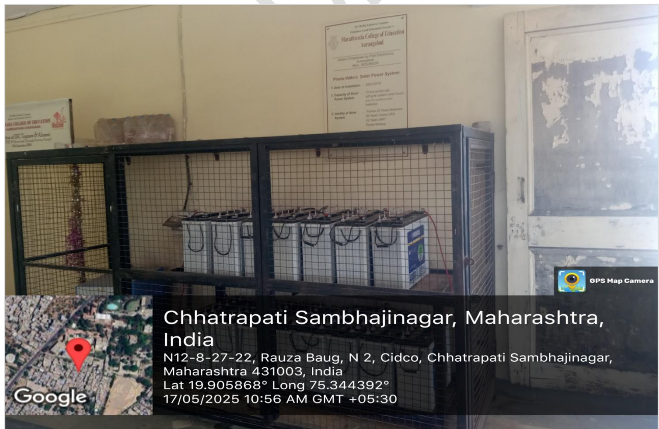
Plate 4: Batteries near the rooftop solar panels
